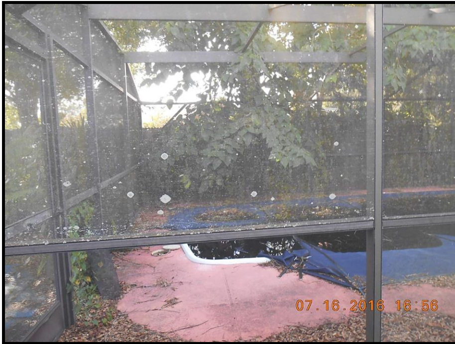
Caption: This Bank of America foreclosure in a Latino neighborhood in Orlando, FL, has an unsecured pool area. Dirty standing water on the pool cover and inside the pool makes a perfect breeding ground for mosquitoes.
